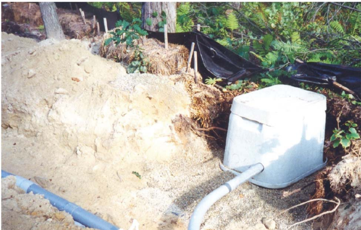
17.0-4 Properly Completed Transformer Installation (Final Grade)
